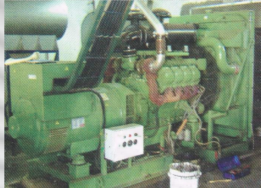
GENSET (MESIN, FAN, RADIATOR)
