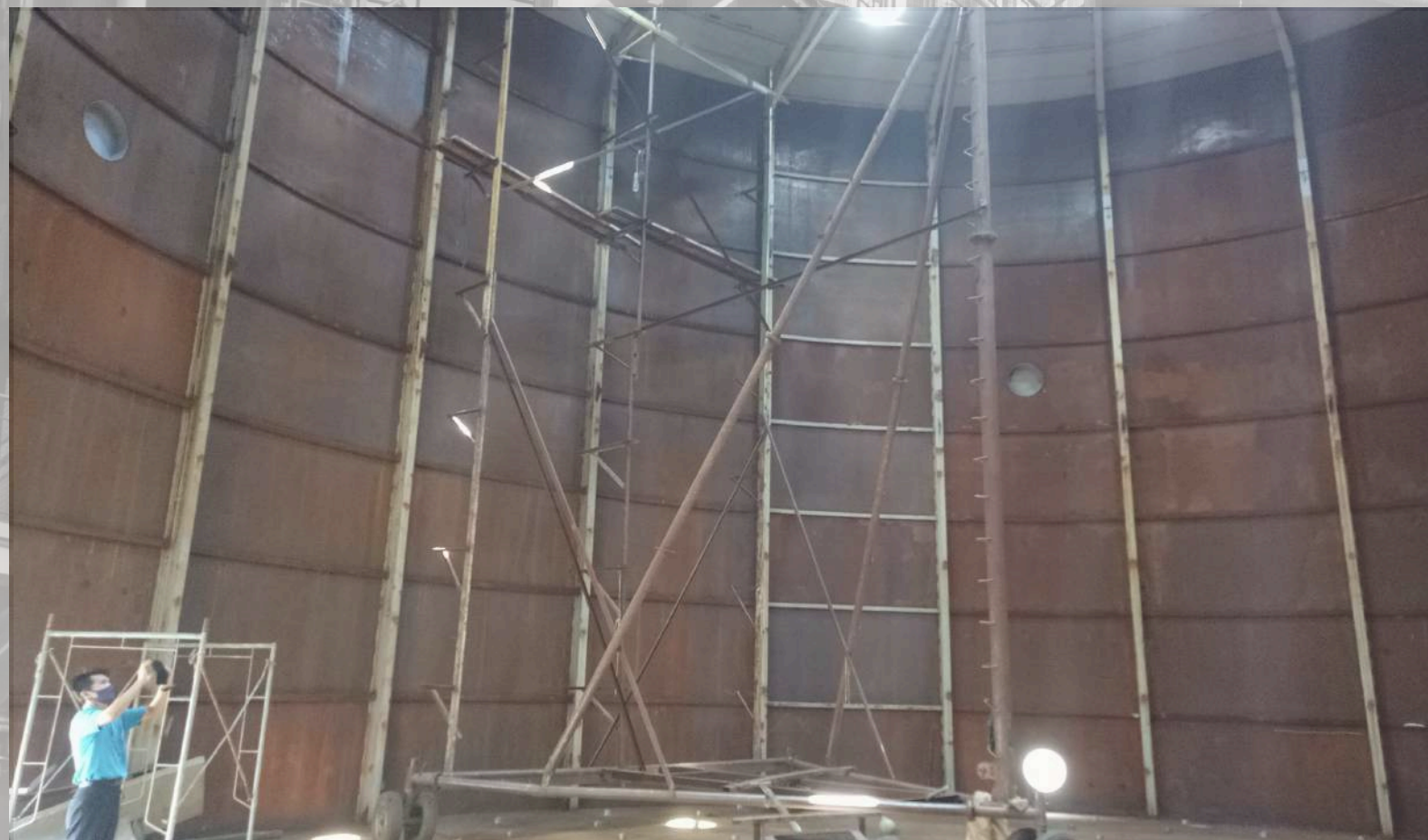
WASTE MANAGEMENT TANK
